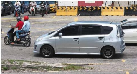
Motorists want Klang Municipal Council to rebuild the damaged concrete dividers along Jalan Langat.
